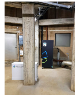
REX installed in reservoirs
