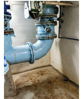
Corrosion on pipes
